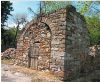
The photo above shows the stone arch and doorway before the stabilization and repointing work was done. Many of the stone were very loose.
