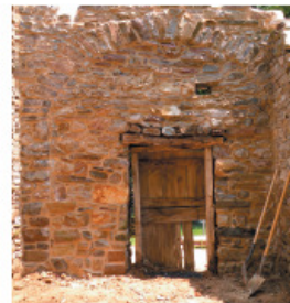
Above: The frame was sinking into the ground.
